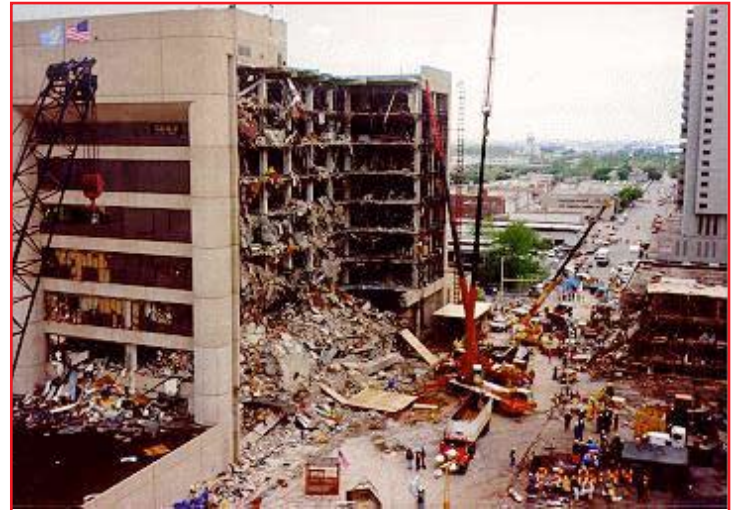
Terrorist bomb damage to Alfred P. Murrah Federal Building, Oklahoma City
