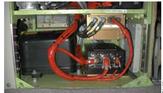
Recorder installed in T-39
